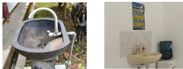
Figure 3. Hand Washing Facilities
