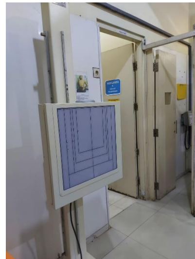
Figure 2. Bucky Stand at the Radiology Installation of Semarang District Hospital
